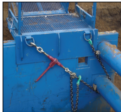
The platform of the Walkway Bridge is securely fastened to the sidewall of the trench shield with an adjustable clamp that fits over the sidewall (far left) and is secured with a ratchet binder.
